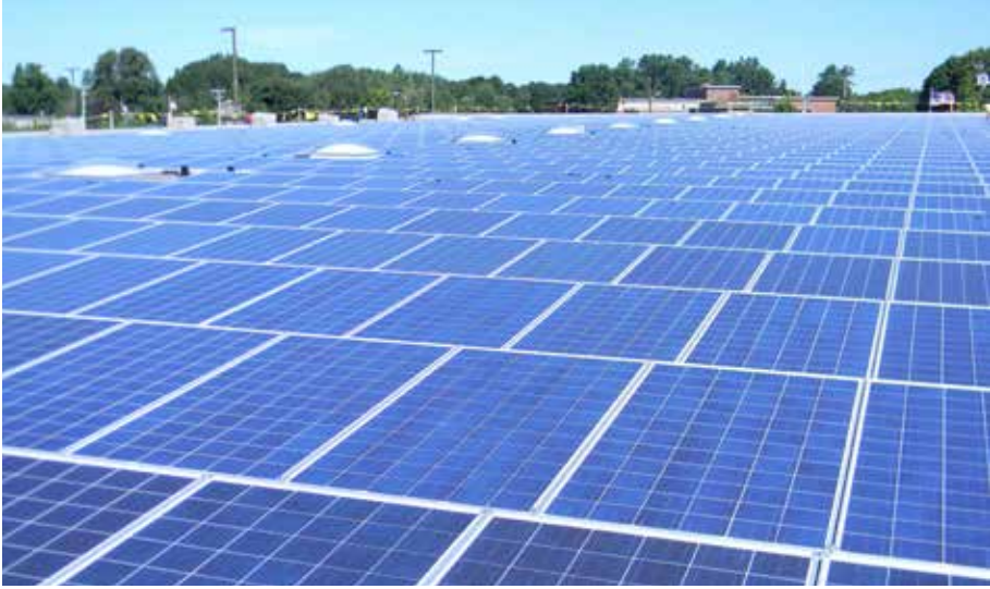
| Solar arrays located at 500 Cummings Center
